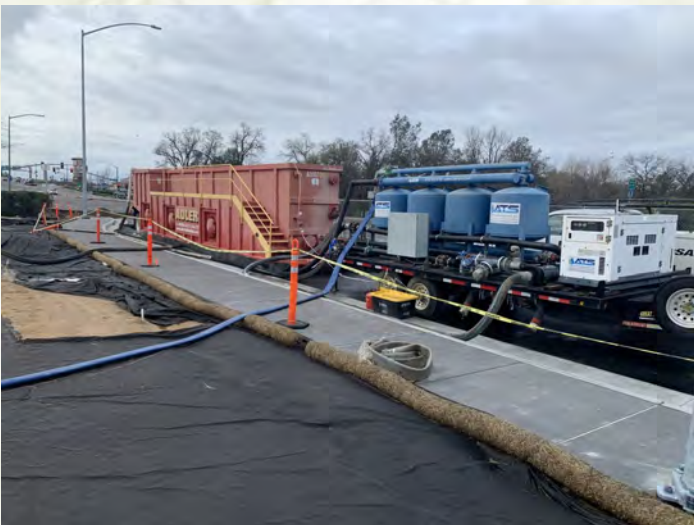
ATS will customize the treatment system to fit your stormwater needs; Pictured: 300 GPM Mobile ATS
